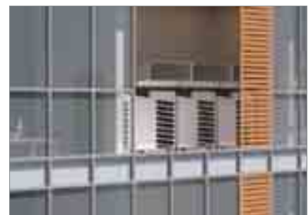
The outdoor unit is hidden inside the building without affecting the overall image of the building
